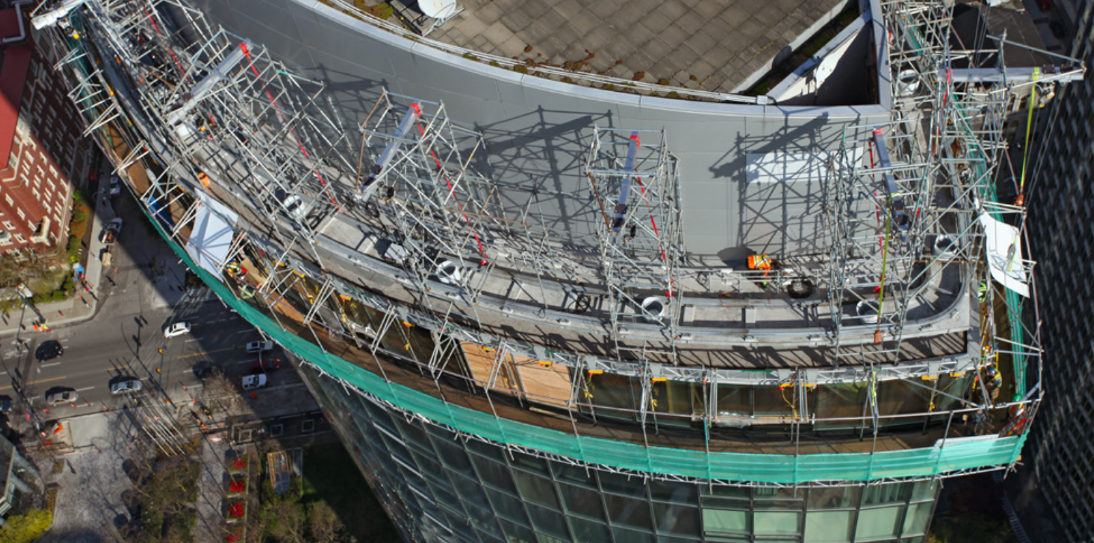
The netting attached to the suspended deck prevents spillage for the One Wall project.
